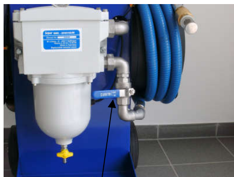
Shut-off valve closed
