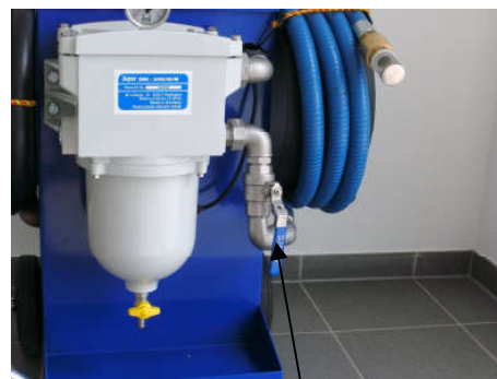
Shut-off valve opened
